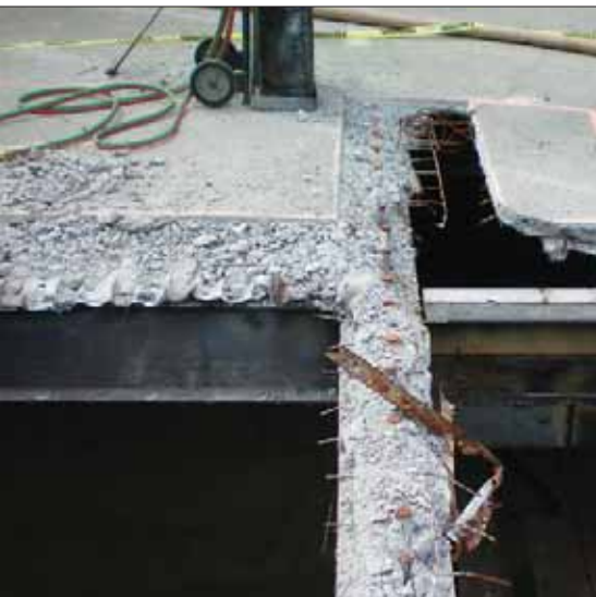
ABOVE: Lack of a maintenance program or deferring maintenance over long periods of time can lead to major structural deficiencies and require costly repairs such as slab replacement.
